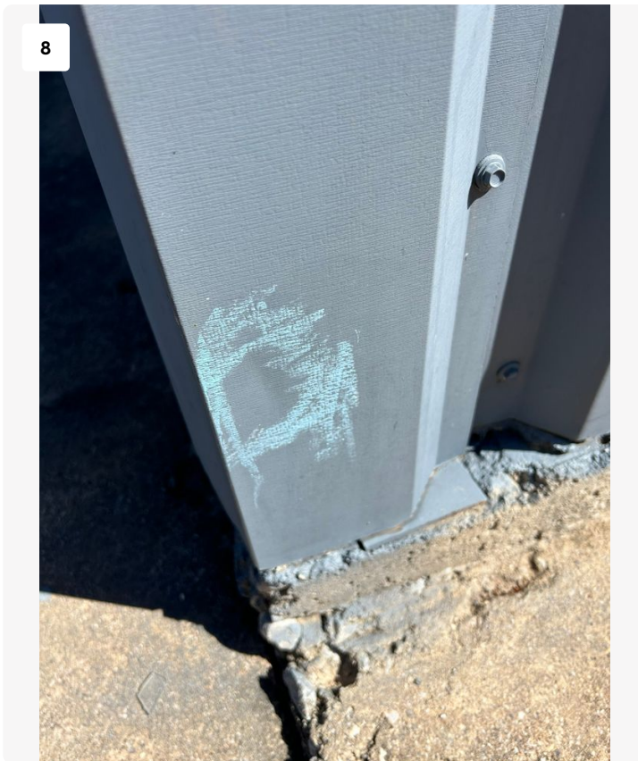
Hail damage to metal exterior wall.
