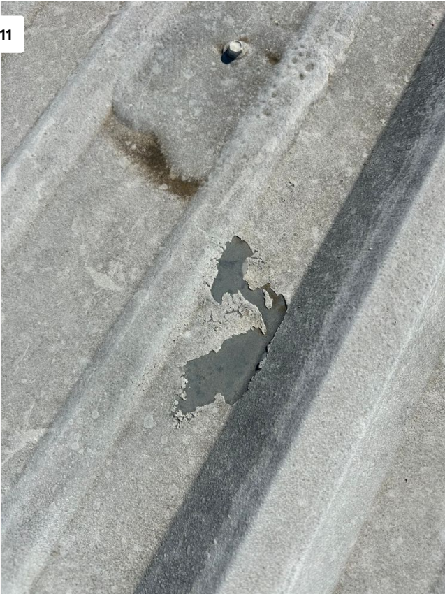
Hail damage Coating has been knocked off of panel.
