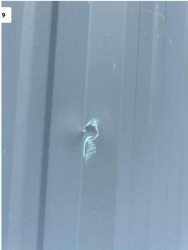
Hail damage to metal exterior wall.
