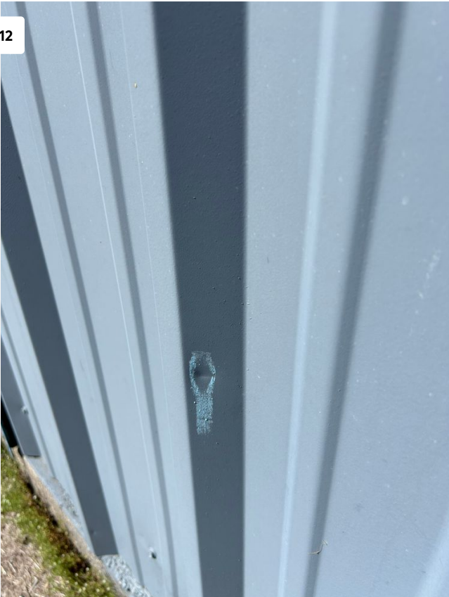
Hail damage to metal exterior wall.
