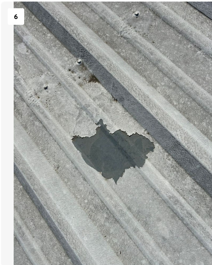
Hail damage Coating is completely knocked off.
