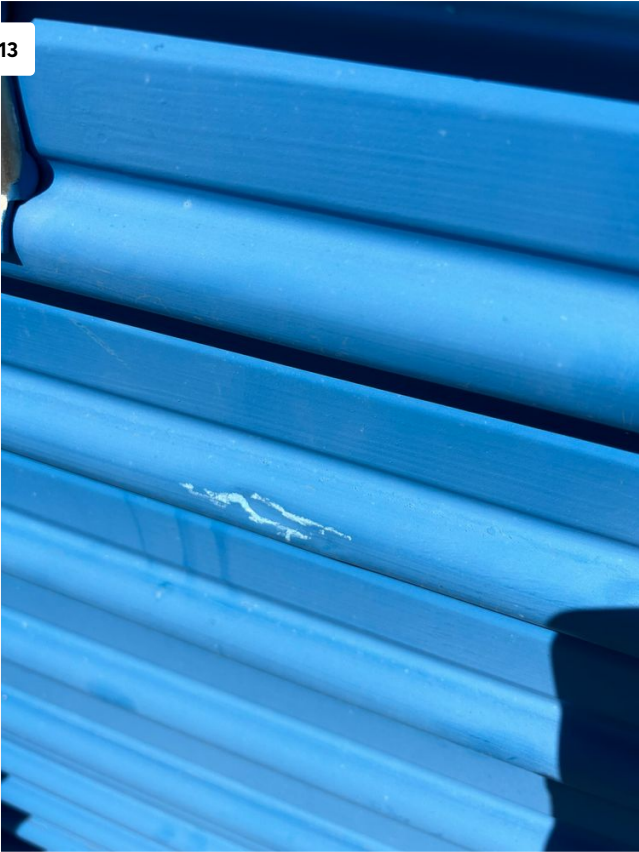
Hail damage to storage door.
