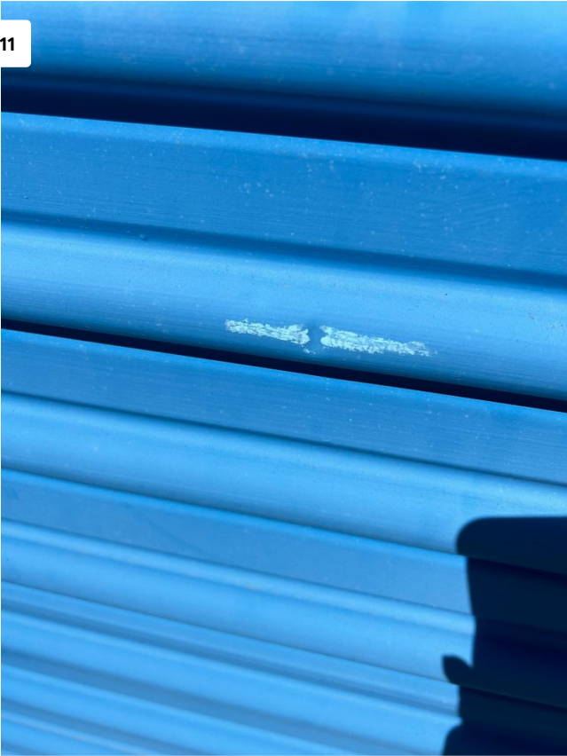
Hail damage to storage door.
