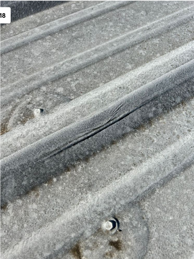
Hail damage to coating which in time will break down and expose the metal panel and lead to a leak down the road.
