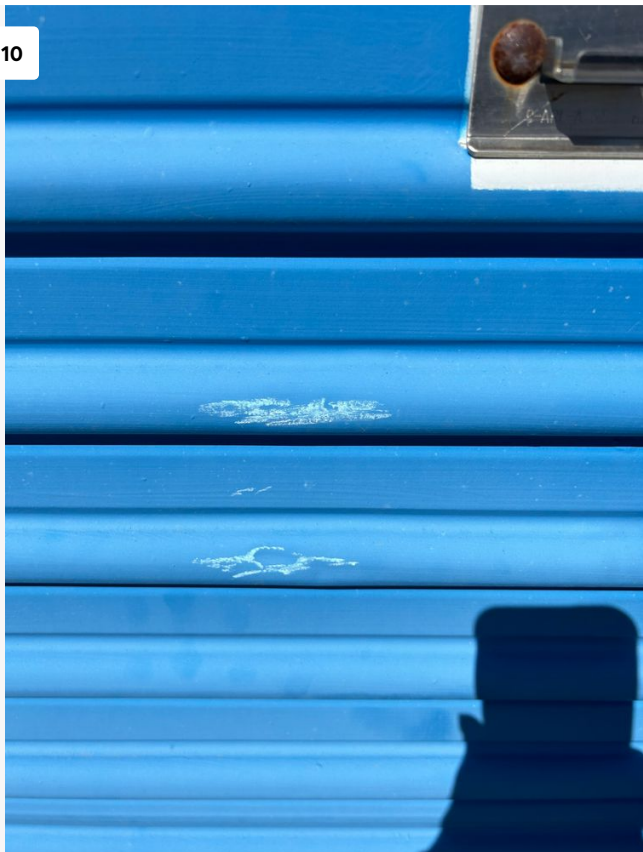
Hail damage to storage door.
