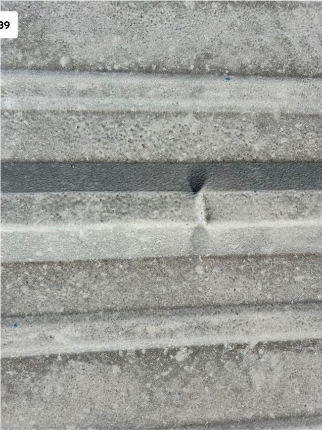
Hail damage or wind driven debris.
