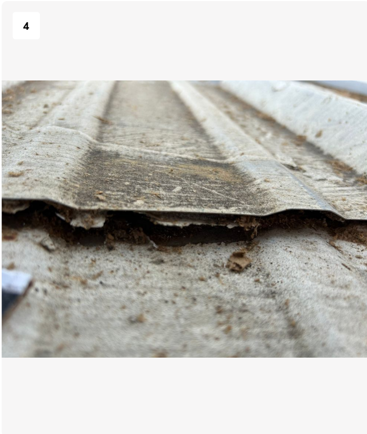
Nestled amidst the orderly array of roof panels lies a subtle but consequential irregularity. Here, where precision should reign, a deviation in alignment has emerged, signaling a potential pathway for water intrusion.
